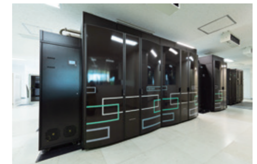
Supercomputer (HPE SGI8600) <Specification> 660 CPU nodes, 26,400 CPU cores Processing speed: 2.02 PFLOPS
