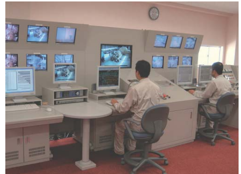
Automatic monitoring and control system for short-circuit testing
