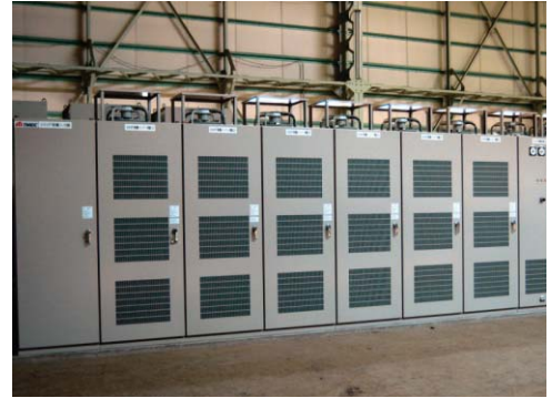
Short-circuit generator frequency conversion system (inverter system)
