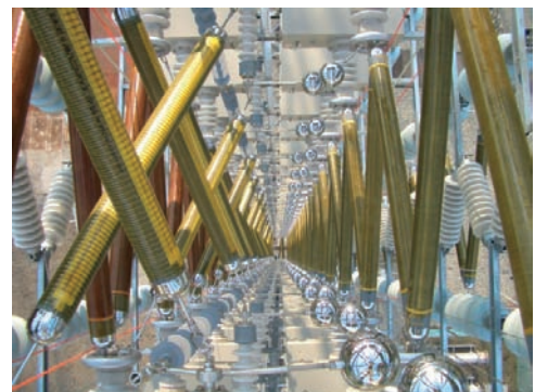
Internal structure of impulse generator
