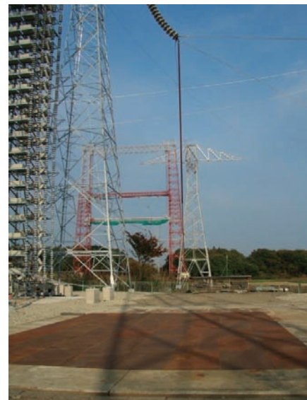
Arrangement of examination that uses impulse generator
