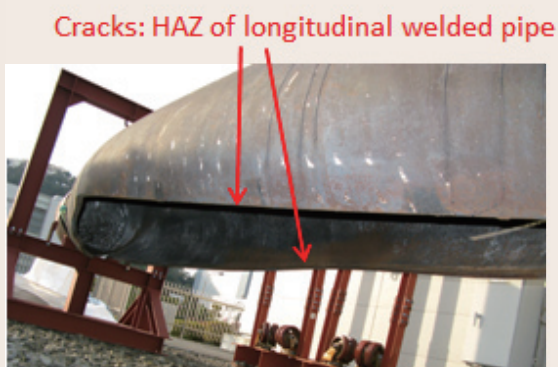
Fig. 5: Photograph of a ruptured 9Cr steel pipe with the dimensions of the actual equipment
