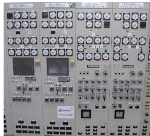
Generator operation panels
